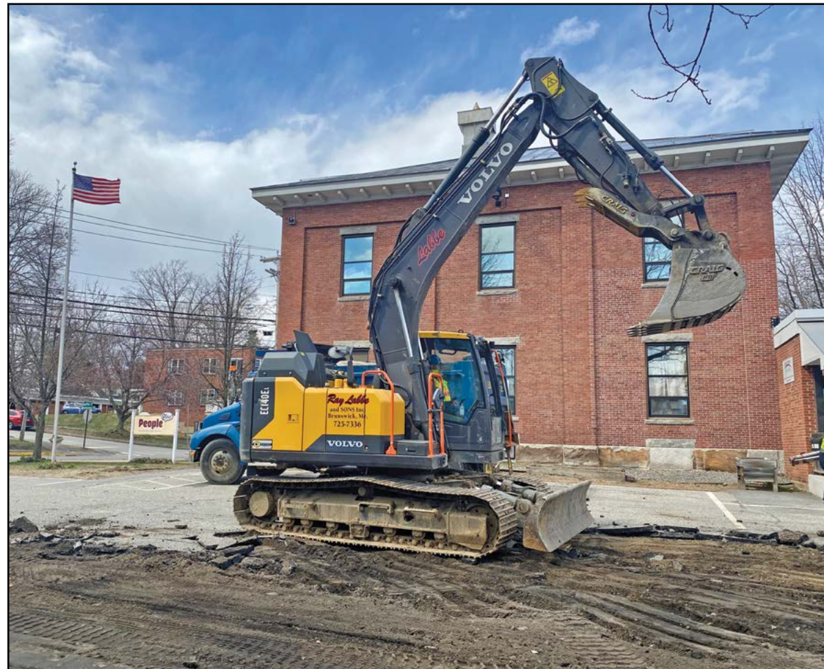
THE PEOPLE PLUS PARKING LOT at 35 Union St. was last constructed nearly 20 years ago and was beginning to show signs of deterioration, including settlement causing puddling during rain events and icing in the winter months. According to Ryan Barnes, Town Engineer of Brunswick, the current project includes the replacement of the existing paved surface, installation of a closed-drainage system, and a new raised sidewalk adjacent to the building. Also, the existing pavement between the trees along the edge of the parking lot is being removed and replaced with loam and seed to help protect the trees in the future.
